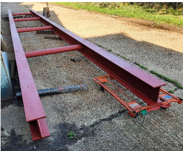
The steel framework that will connect the two sides of the stream and itself support the bridge deck and sides (to a design by Chris Cuff).
