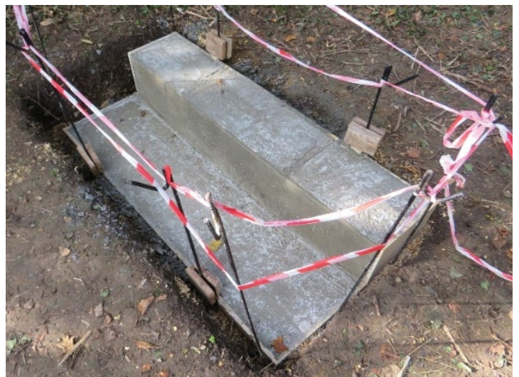
The westernmost of the 'L' shaped footings that between them will support the bridge superstructure.
